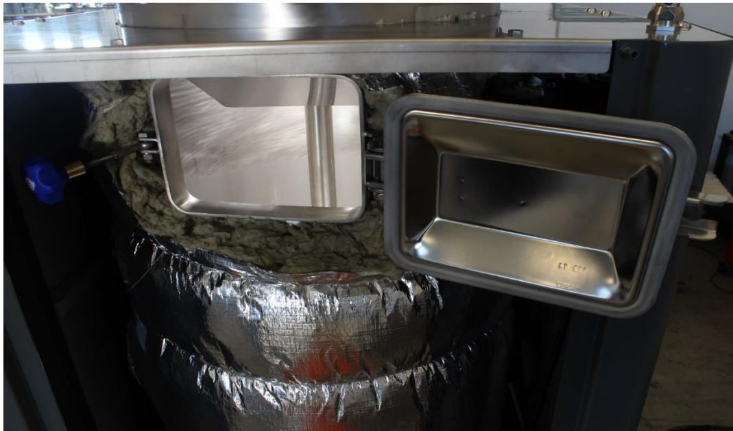
Inner tank inspection door
