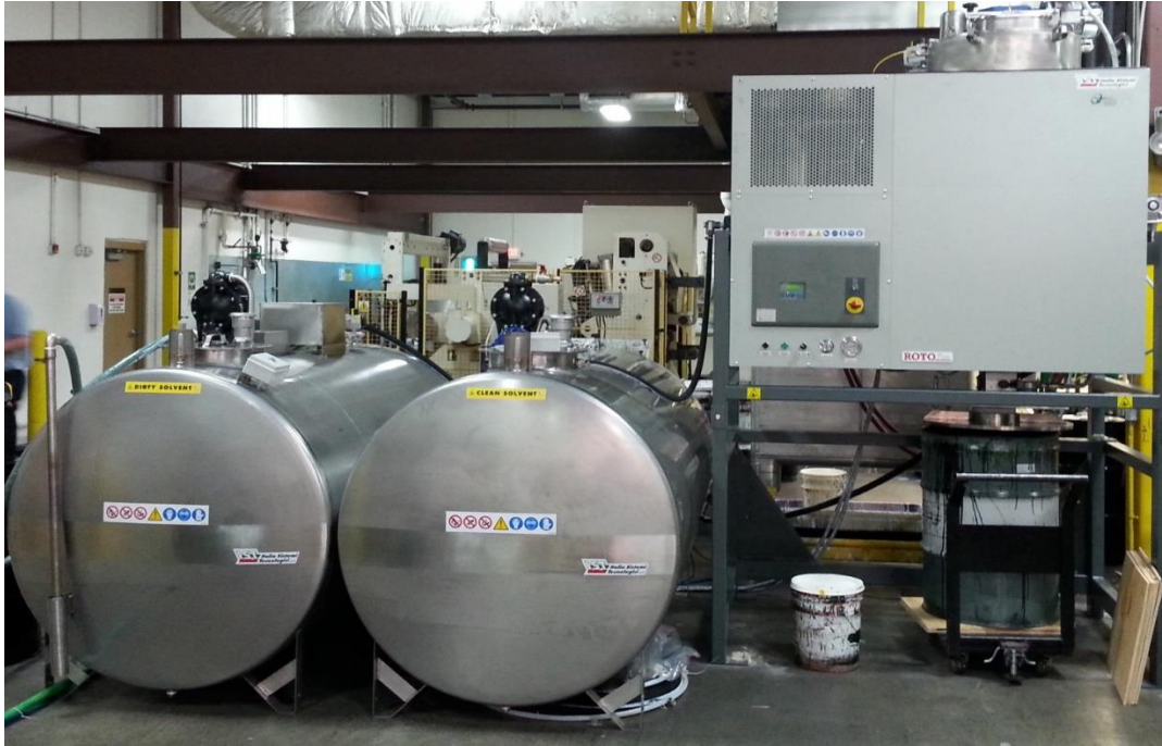
Stainless steel solvent tanks
